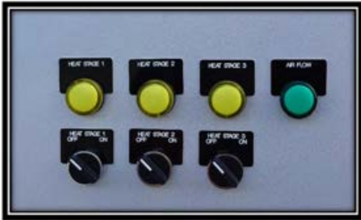
(Close up of Control Panel)
